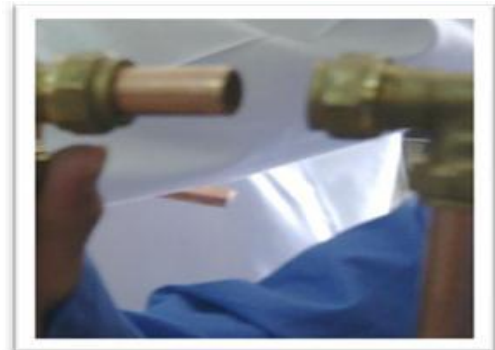
Figure 4- Pipe connected with T-function
